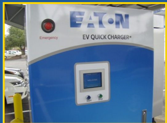
Eaton DC Fast Charger
