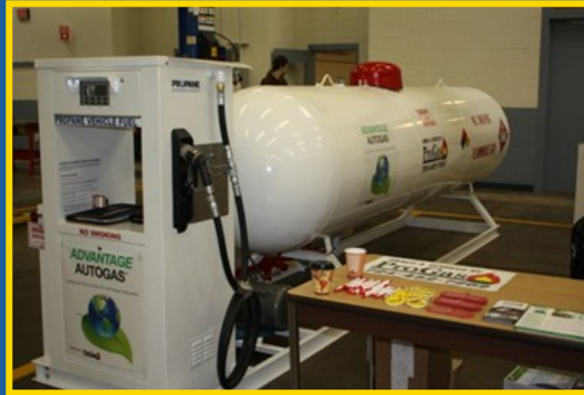
Pro Gas Propane Refueling Station
