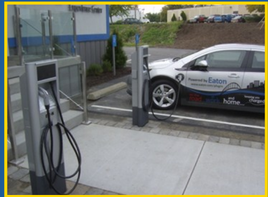
Eaton Level II Chargers at Warrendale, PA
